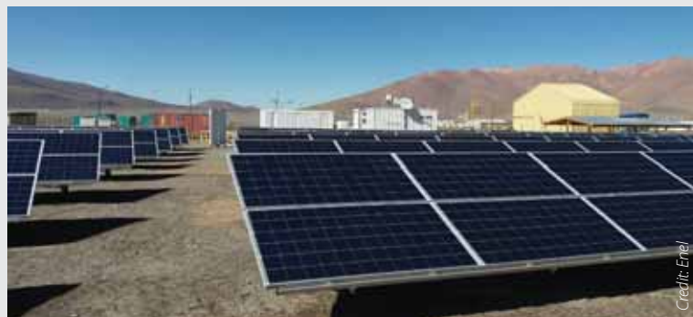
Enel's "plug-and-play" commercial-sized micro-grid powered by solar PV together with hydrogen and lithium storage.
