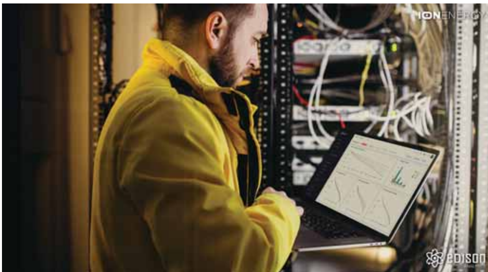
ION Energy won a deal to work across esVolta’s portfolio after “showcasing the value” and “material impact on the ROI” that its Edison Analytics platform could have.
