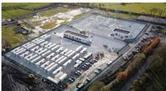
Credit: Lumicon Energy Storage
